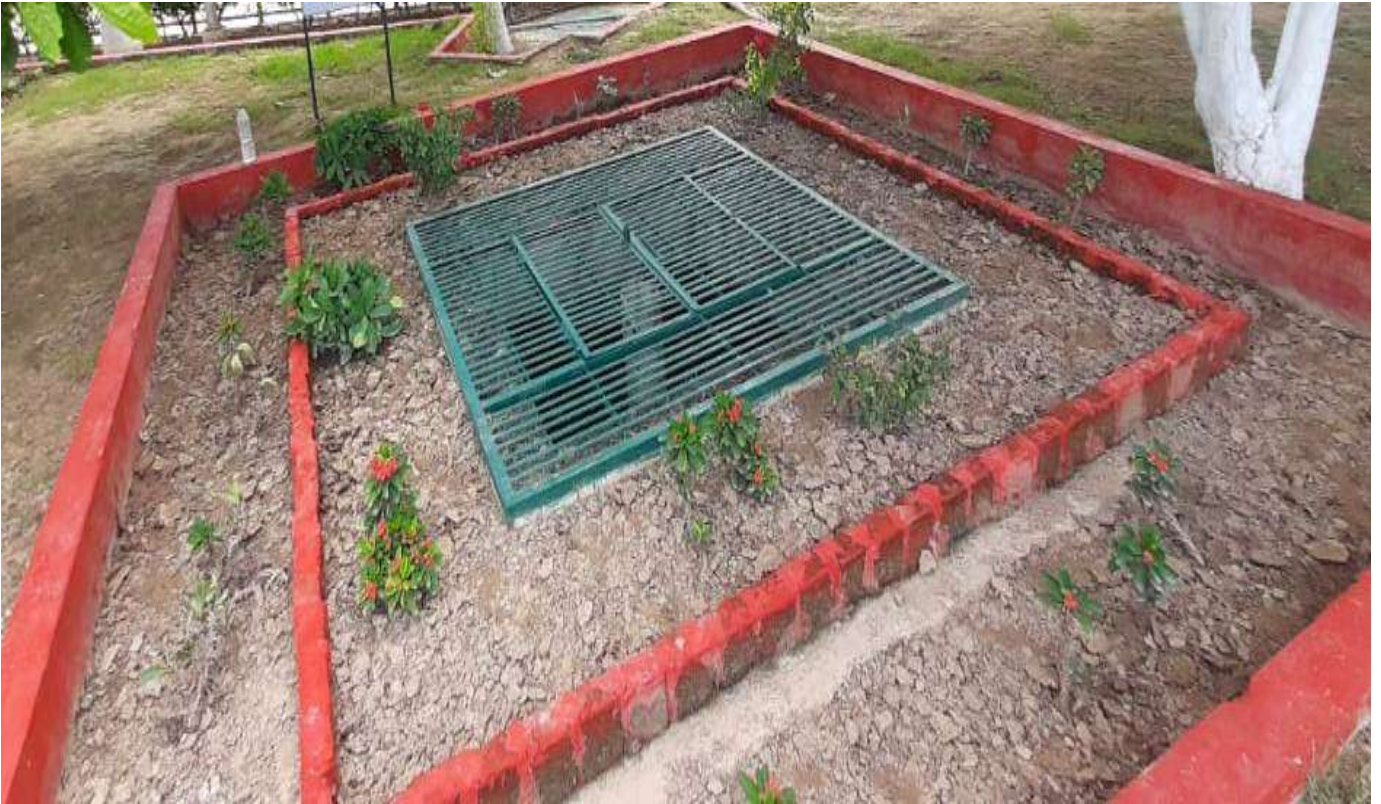
An Example of Rain Water harvesting underground well which may be constructed in GSC, Naya Nangal Campus
