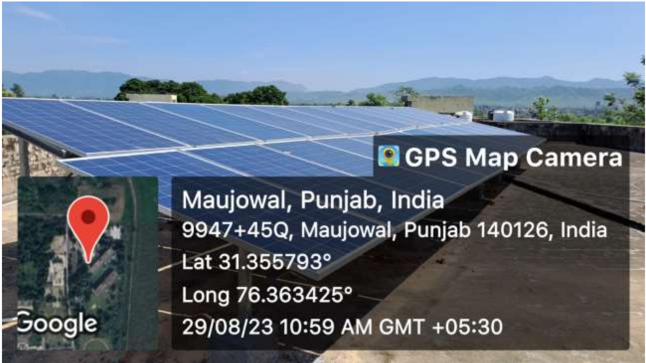
Grid connected Solar PV Plant installed in Govt. Shivalik Campus
